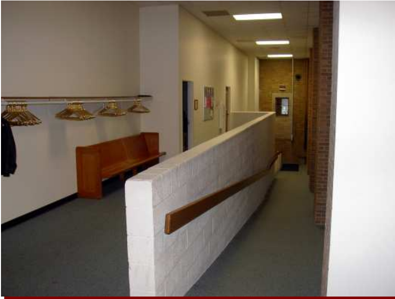
View of the new Ramp Access to the Main Floor and the Basement.
